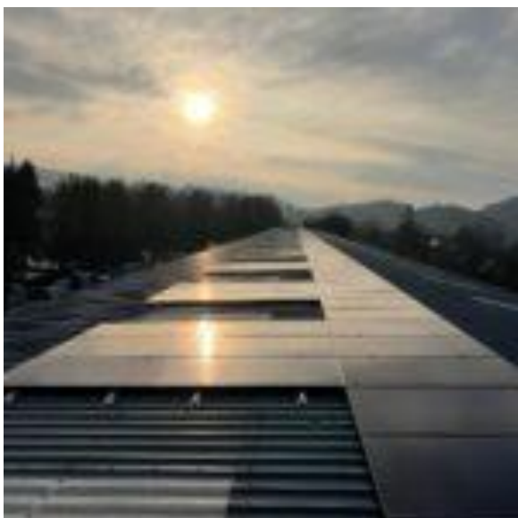
Hornsey Steel Rooftop Solar Panels
